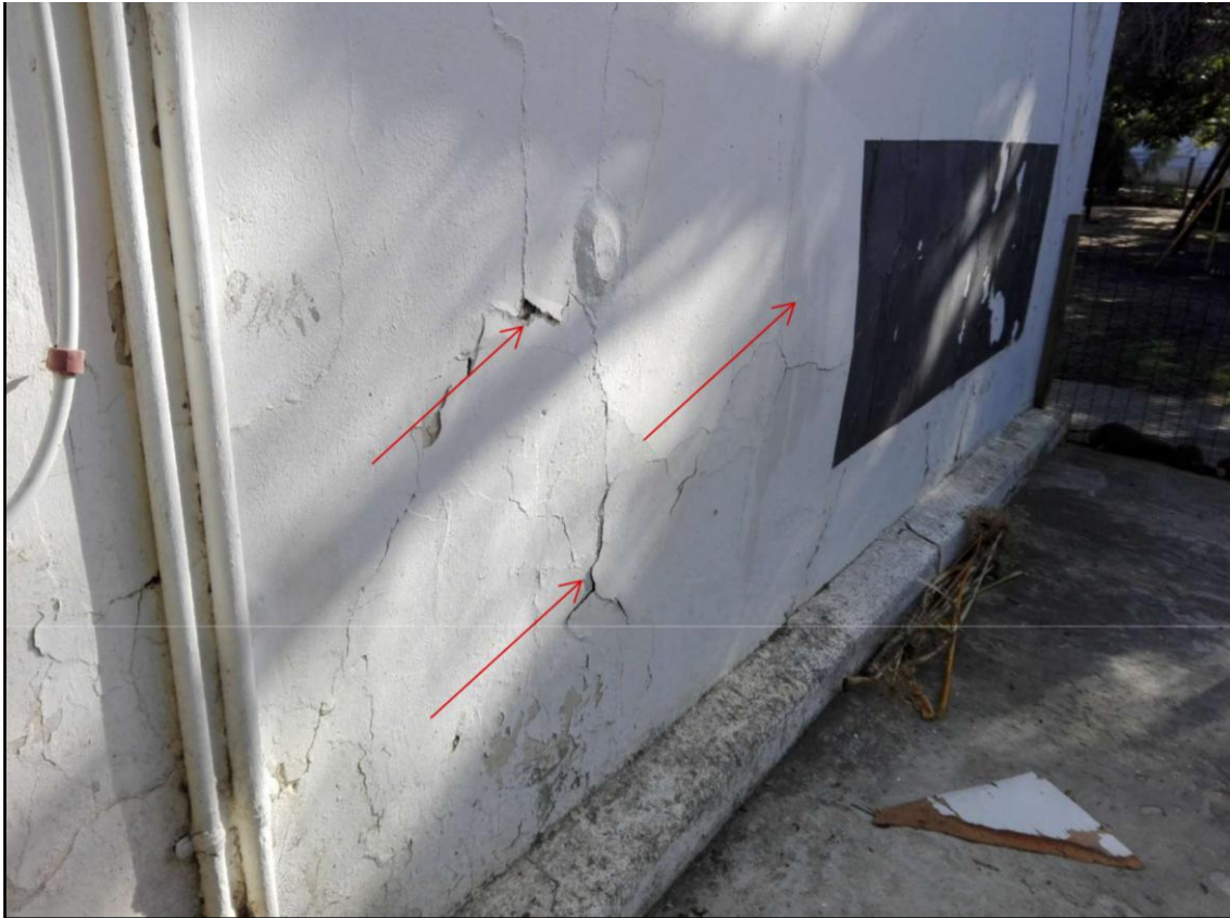
Figure 8. Plaster at northern end of building failing due to moisture seepage.
