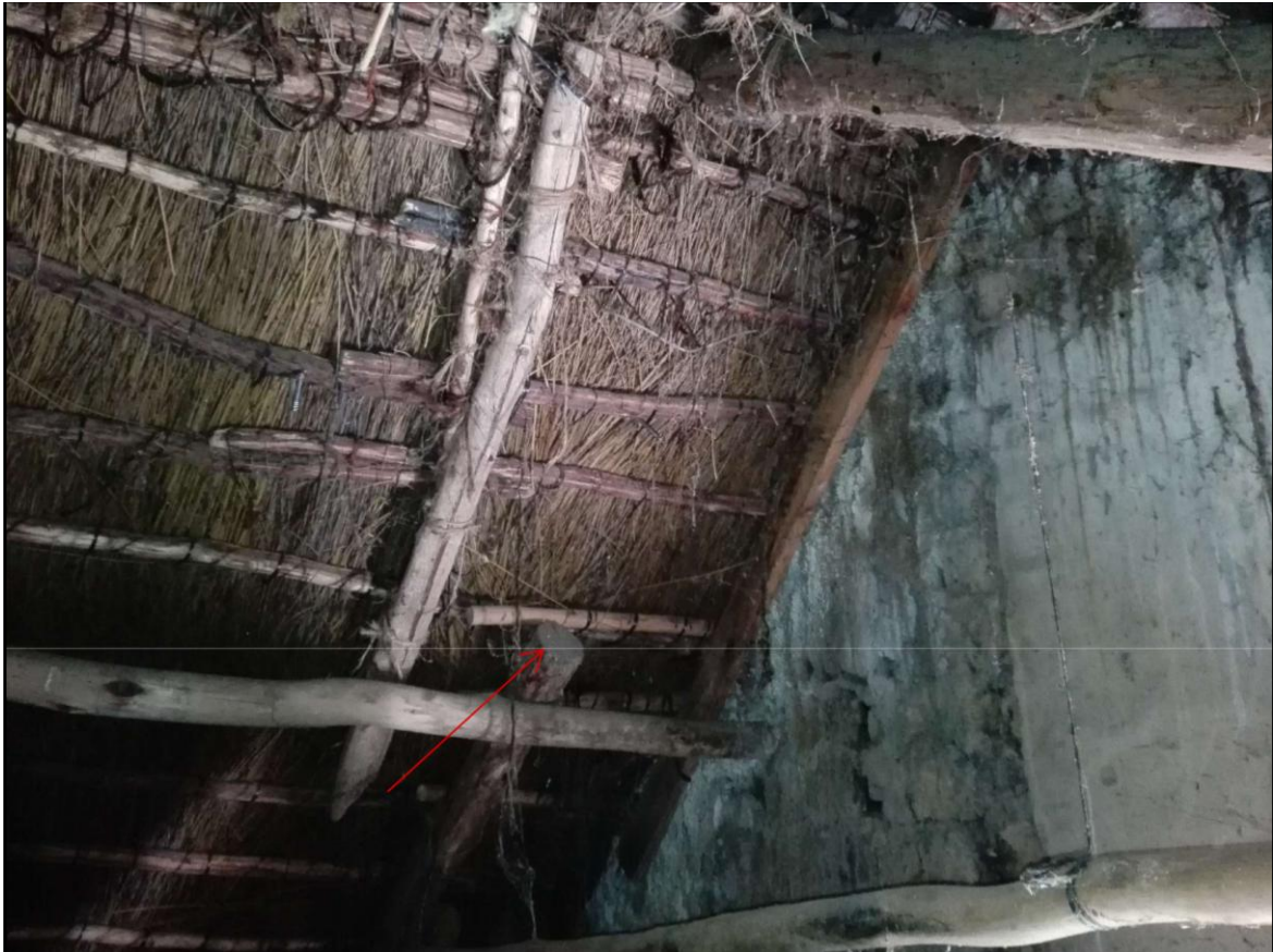
Figure 3. Truncated rafter at northern end of building.
