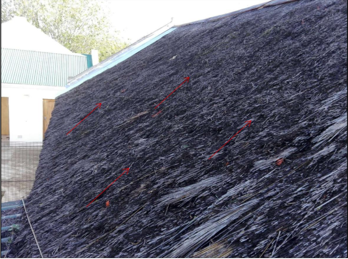
Figure 5. Degraded thatch to be replaced or patched.
