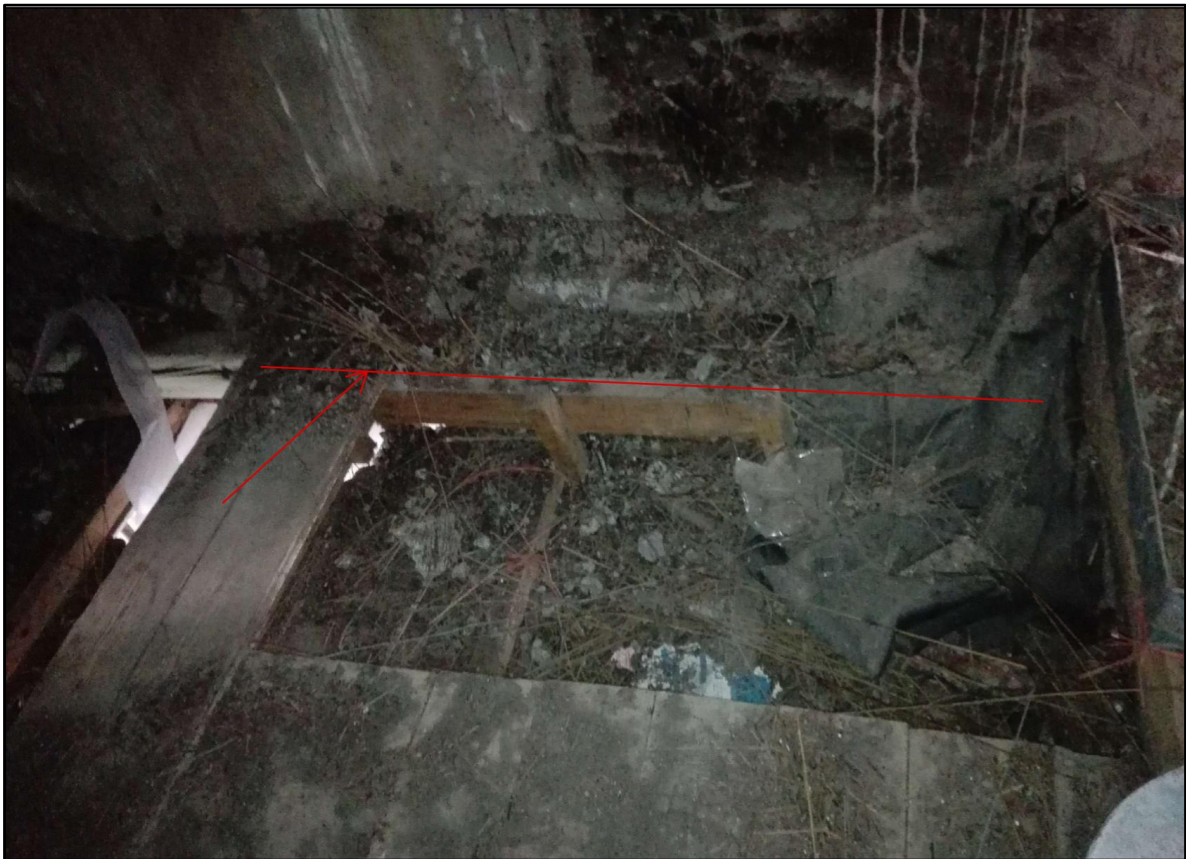
Figure 1: Truncated tie beam at northern end of building where original fireplace was located.
