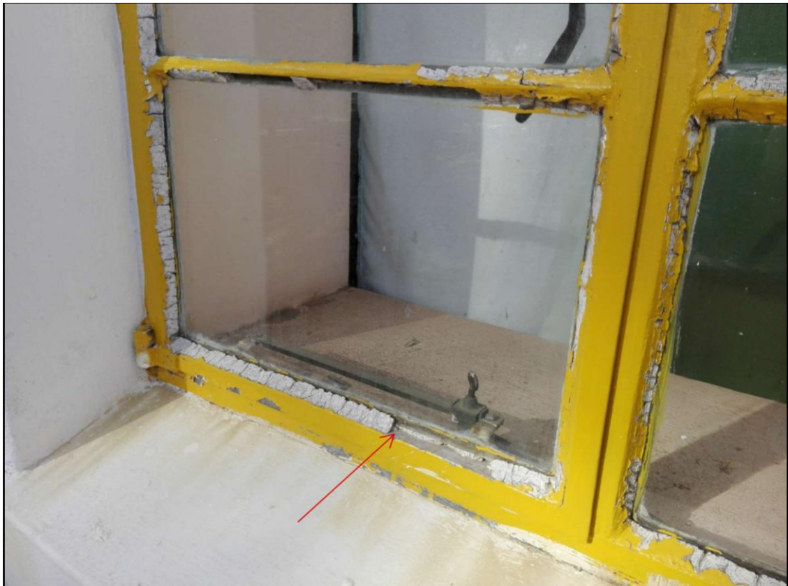
Figure 9. Metal frame windows in poor repair.
