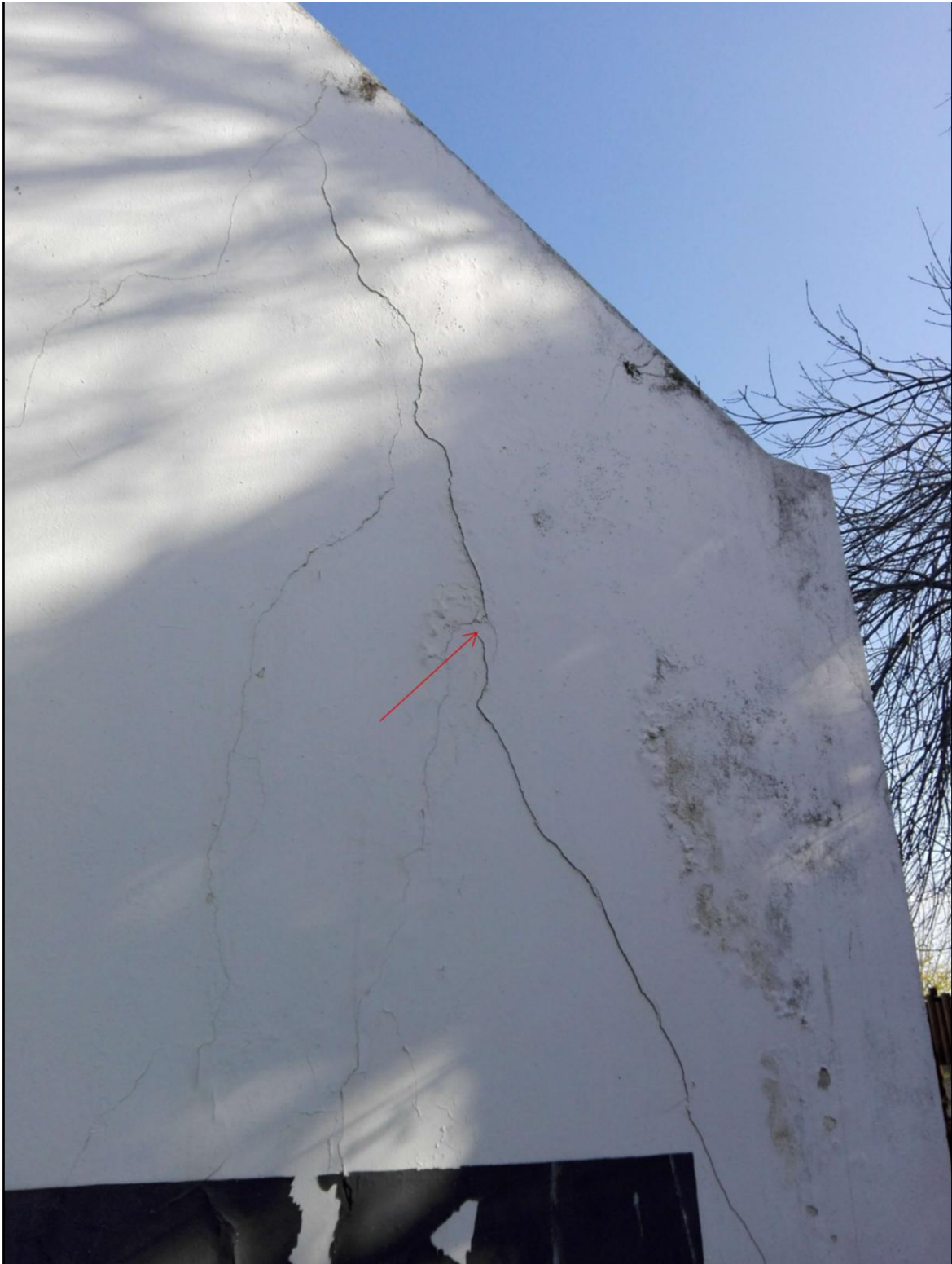
Figure 7. Cracks in plaster at southern end of building requiring repair and repainting.
