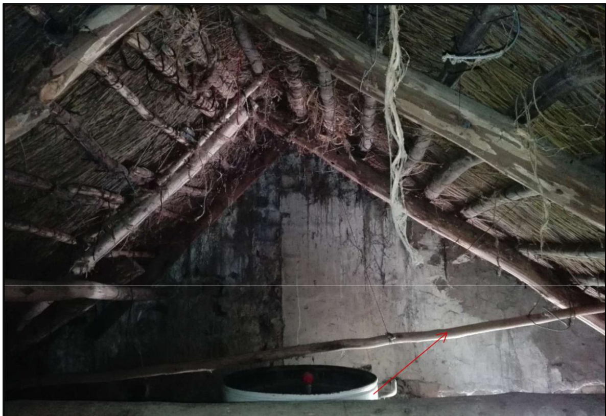
Figure 2. Damaged collar tie at northern end of building. Blackened plaster shows location of original chimney.
