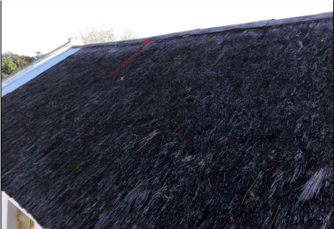
Figure 6. Metal ridge capping to be replaced with cement/plaster capping.
