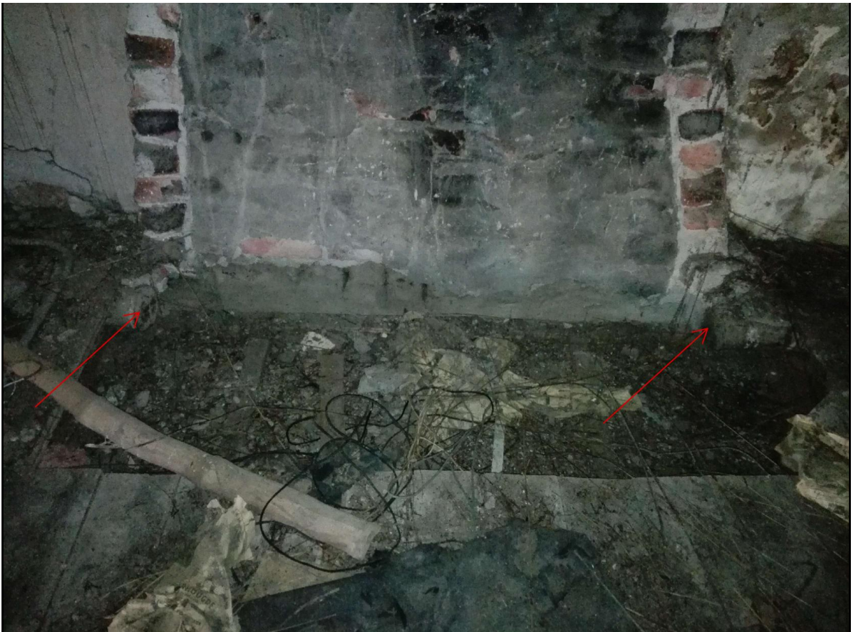
Figure 4. Truncated tie beam at southern end of building. Brick-built chimney of later fireplace visible.
